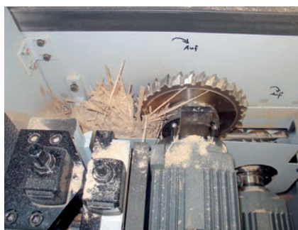
Broken splinters block the extraction hood - fire risk through friction of the rotating tool!
